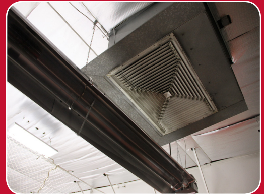
HVAC systems & equipment optimization
