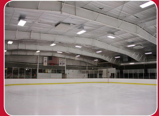
Comprehensive lighting retrofit with T5 lighting improved quality of light and saved energy.
